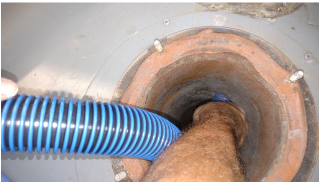
Hose Inserted into Swirl Tube Heat Exchanger
