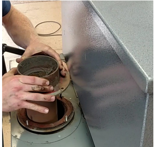
Lifting Out the Flue Tube Assembly
