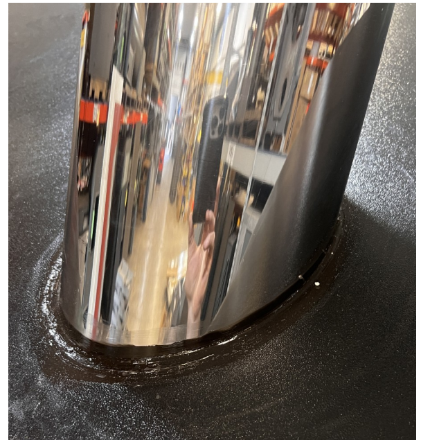
Silicone Seal where Insulated Flue Pipe comes through the Roof
