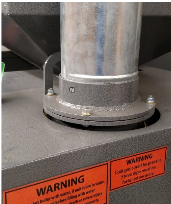
Flue Pipe Connection
