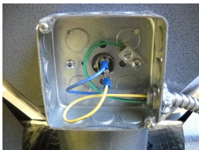
Hopper Temperature Safety Switch: Cover Open
